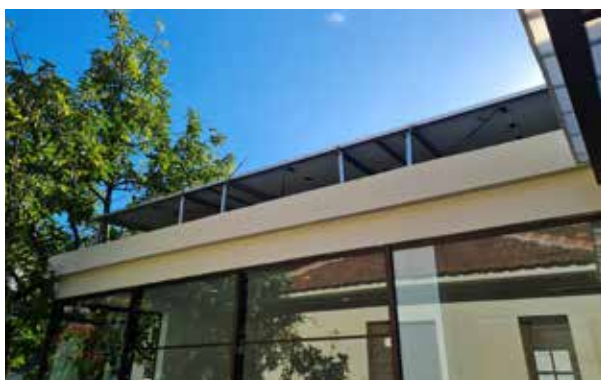
Patio House - Solar Panels
